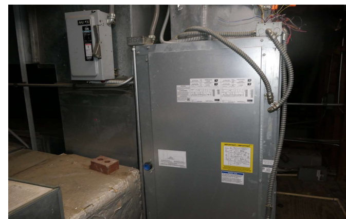
Newer split system unit serving the cafeteria.
