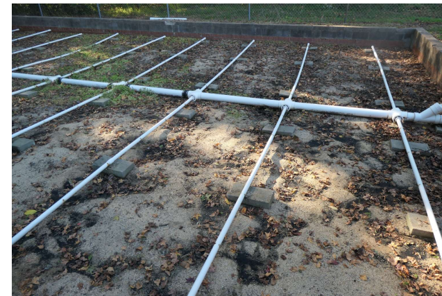
Overview of the sand filtration bed for the septic system.
