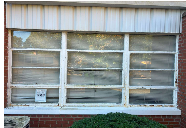
Single pane windows are in poor condition.
