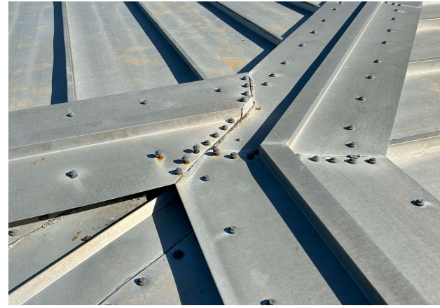
Failed fasteners/gaskets noted at the metal roof.
