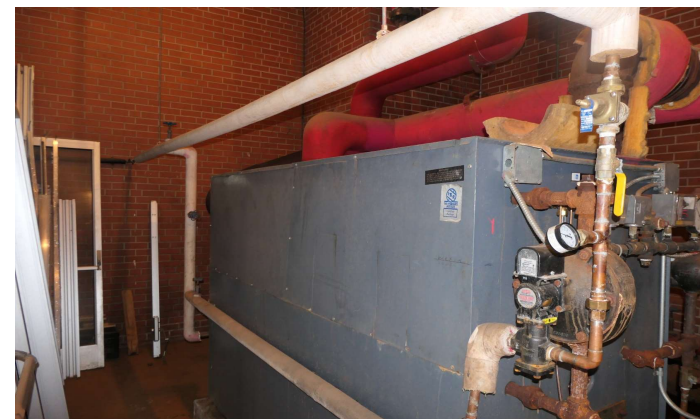
Steam boiler and heat exchanger for hydronic heating.
