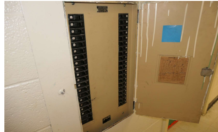
Typical obsolete electrical equipment.
