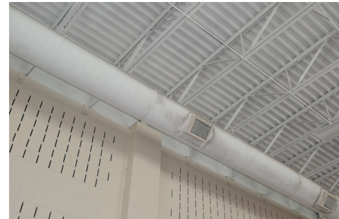
Dust/debris noted on the ductwork of the gymnasium.
