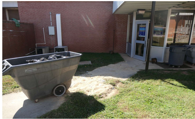
Area of poor drainage which enters into the building.
