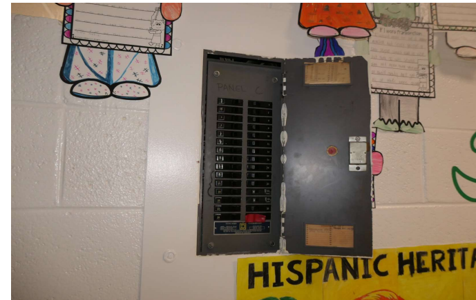
Vintage electrical panel which should be budgeted for replacement.
