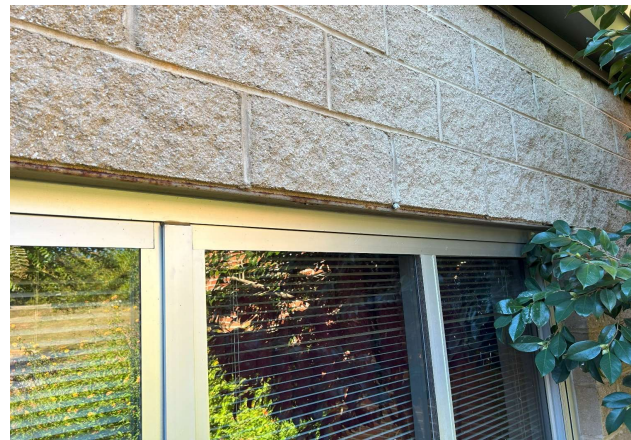
Typical lintel with noted corrosion.
