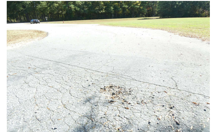
Typical condition of asphalt pavement with alligator cracking.
