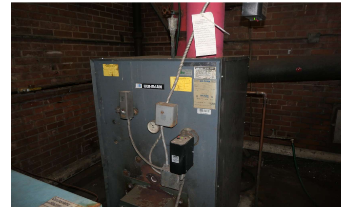
Typical heating hot water boiler.
