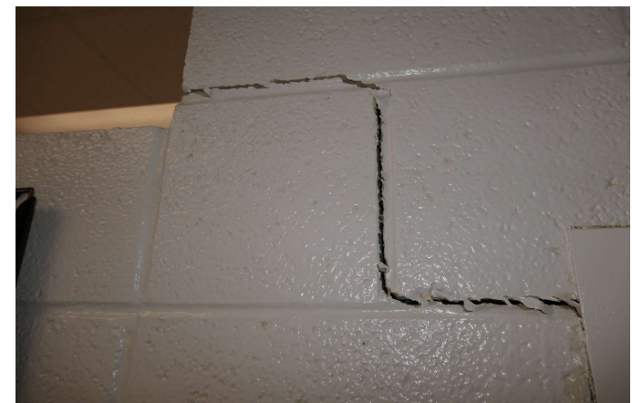
Interior step cracking of a CMU wall.
