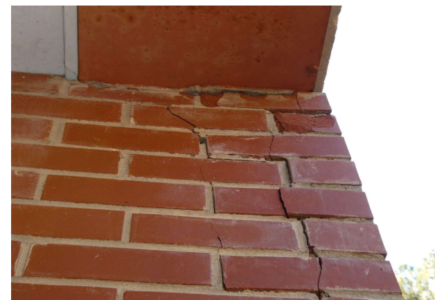
Minor cracking at the amphitheater area.
