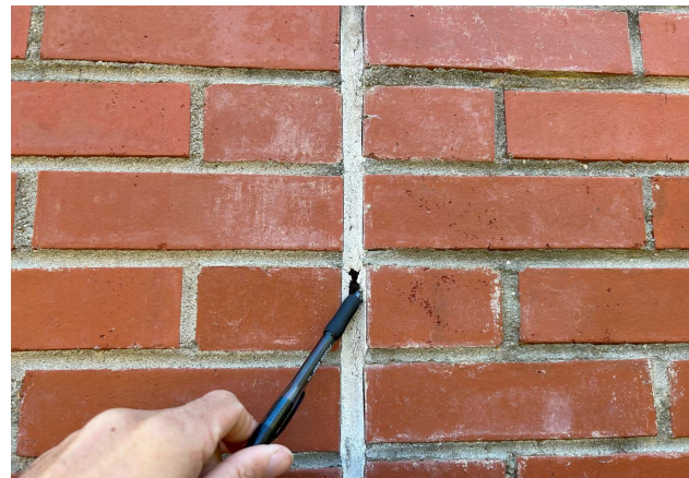
Deteriorated expansion joint sealants
