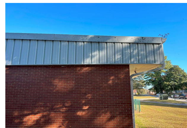
Organic growth on fascia panels.
