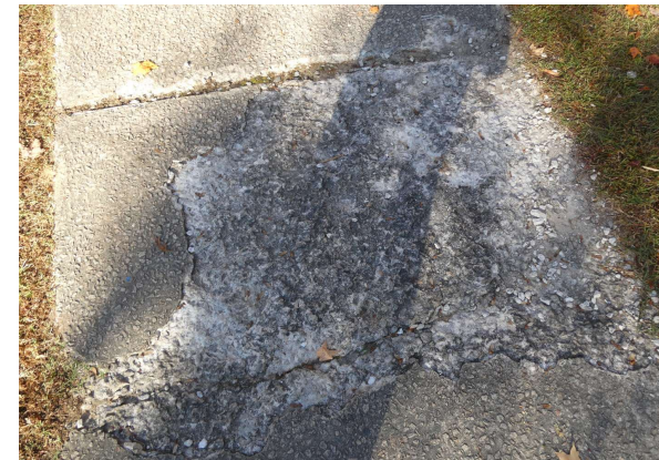
Delamination at concrete sidewalks noted.
