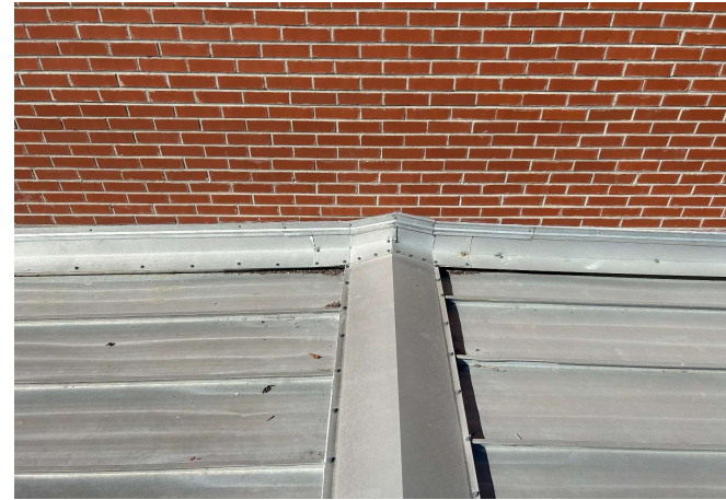
Building transitions have poor detailing.
