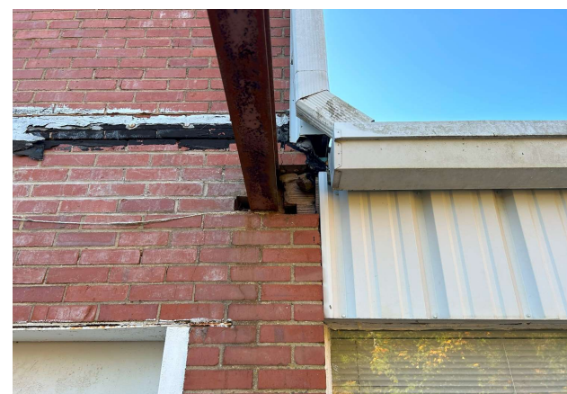
Exposed steel which should be enclosed.
