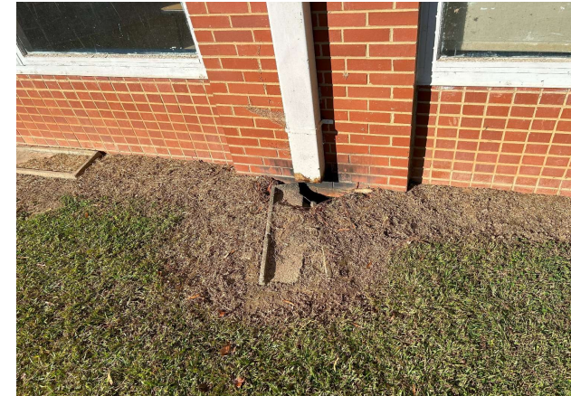
Downspouts not connected to drainage piping.
