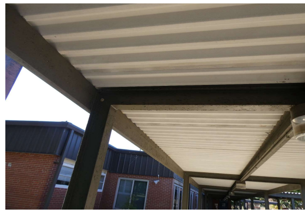
The framing for the covered walkway has evidence of historical corrosion which has been painted over.
