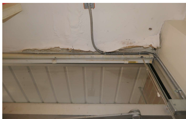
Water ingress due to poor building joint.
