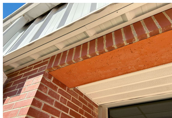
Typical lintel with corrosion.
