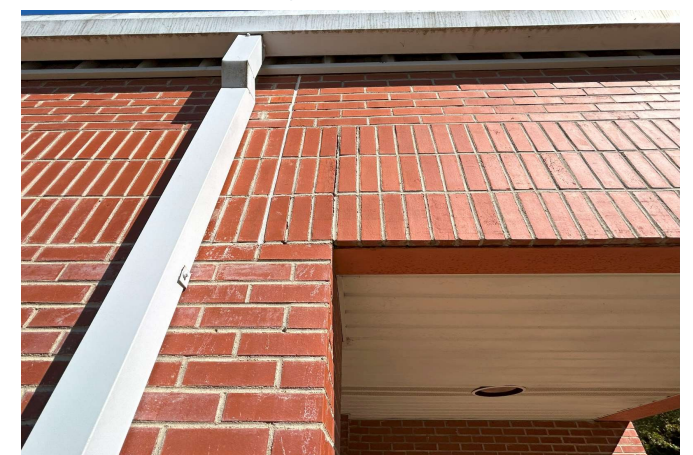
Area of debonded mortar.
