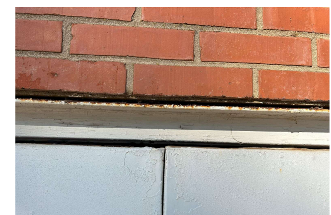
Corroded lintels noted at several locations.
