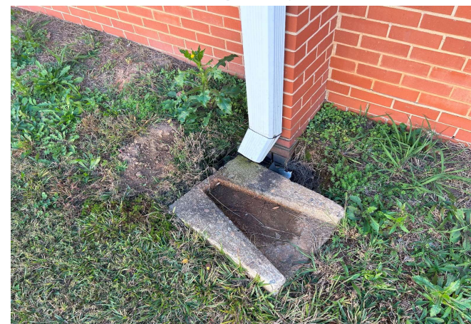
Downspouts don't direct water away from the building.
