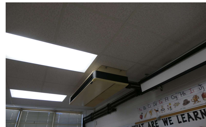
Typical ductless split system serving the classrooms.
