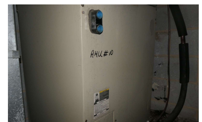
Air handling units are in poor condition.
