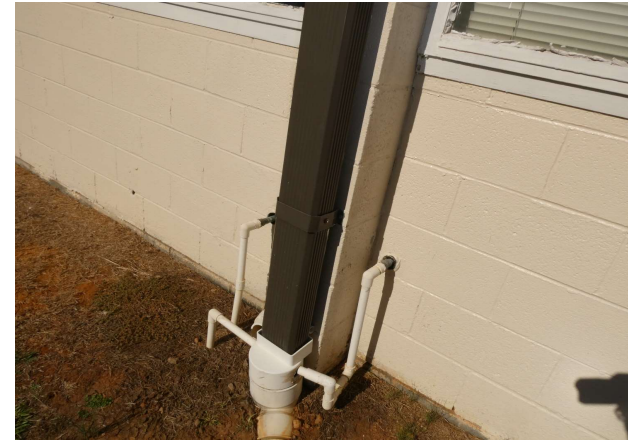
Downspouts are connected to drainage piping.
