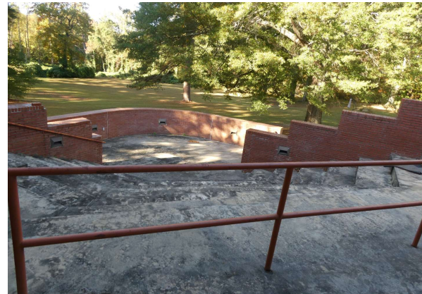
Significant settlement issues were noted at the amphitheater.
