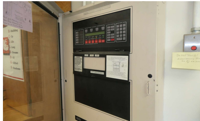
The fire detection and alarm system is obsolete.
