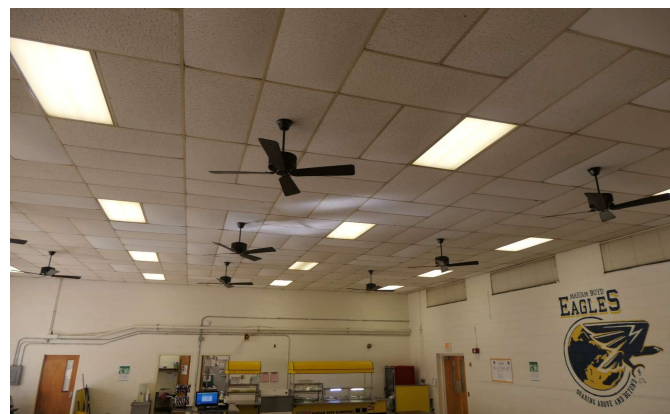
Sagging ceiling tiles often indicate potential humidity issues.
