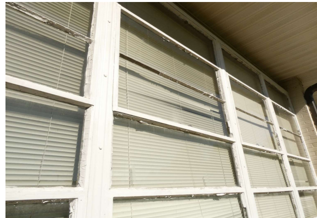
Original windows with noted corrosion and sealant failure.
