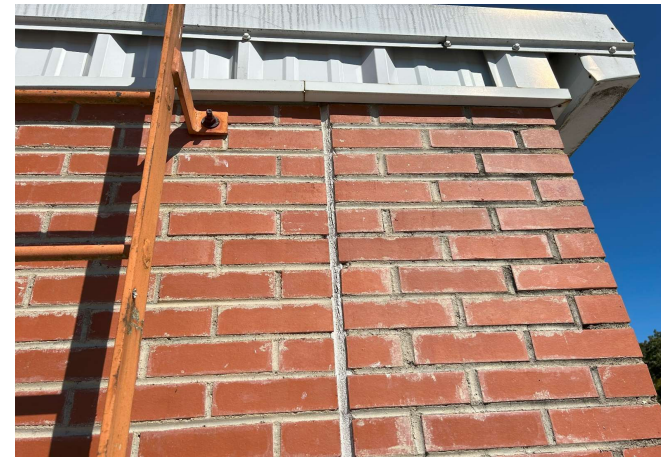
Deteriorated expansion joint sealant.
