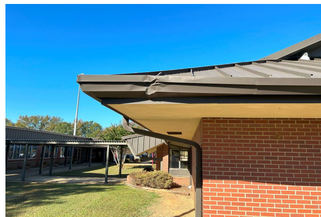
Section of damaged guttering.
