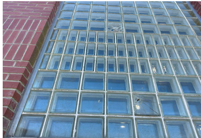
Cracked glass block.
