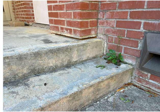
Missing/deteriorated sealants at the base of the walls.
