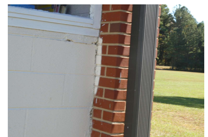
General condition of exterior sealants.
