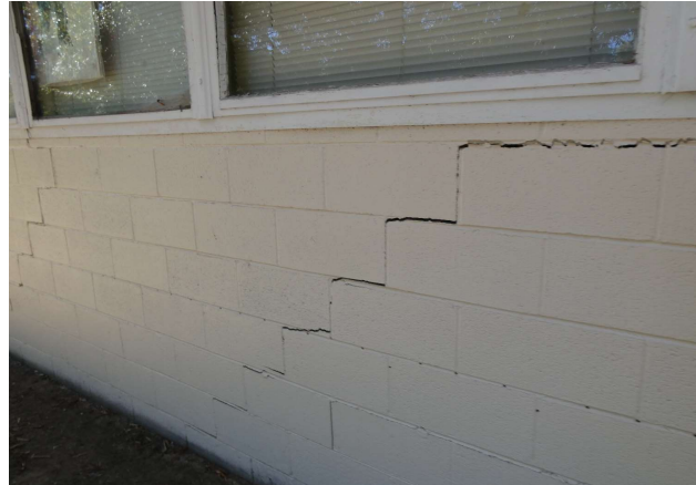
Exterior stair step cracking due to noted structural issues.
