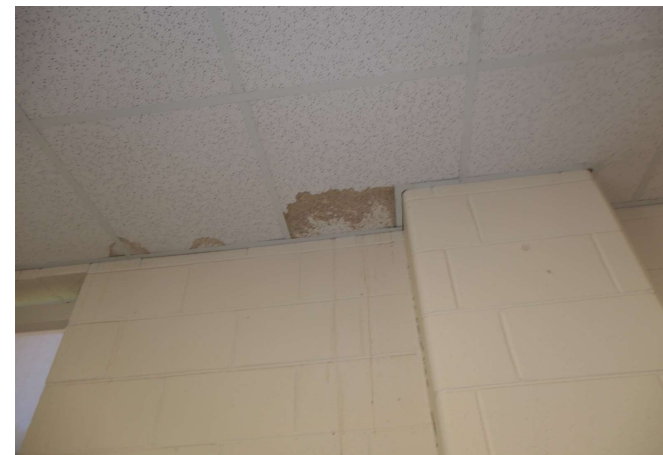
Stained ceiling tile likely caused by roof leak.
