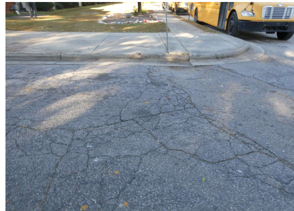
Asphalt with alligator cracking.
