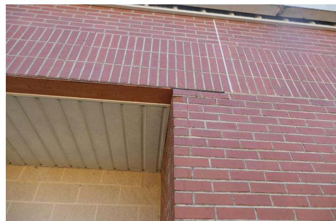
Displaced mortar at one of the lintels.
