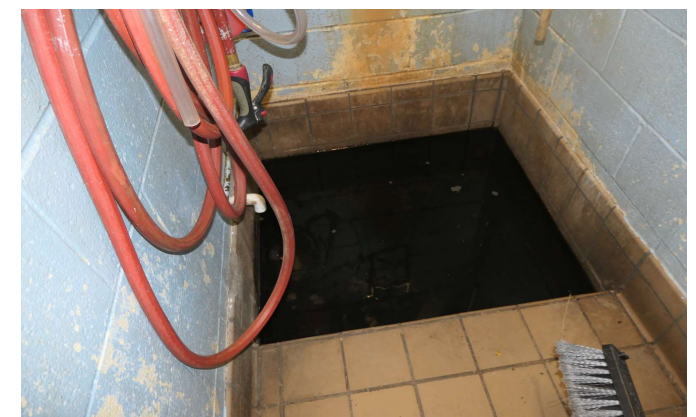
Clogged mop sink drain due to grease trap.
