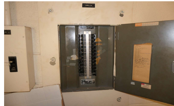
Federal Pacific electrical panels are obsolete.
